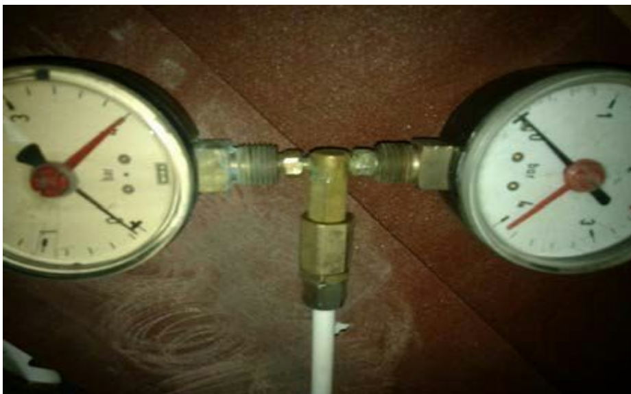
Detail of the connection for the pressure gauges
